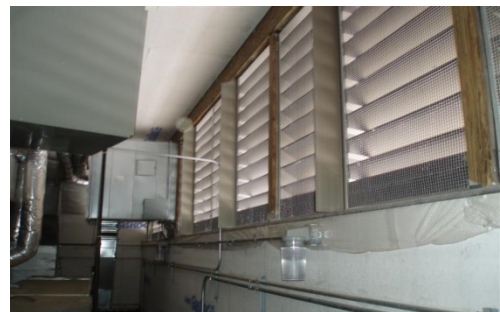
Figure G-48. Outside Air Intake Louvers in the VRF-1 Penthouse.
