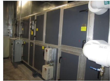
Figure G-7. DV-2 Make Up Air Handler
