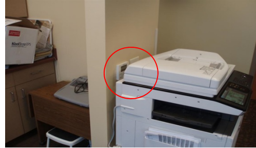
Figure G-49. VRF-1 Thermostat Located Behind a Copy Machine that Emits Significant Heat.
