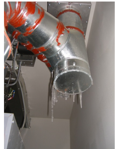
Figure G-68. VRF-3 Freezing Observed on Heater Exhaust Ducting
