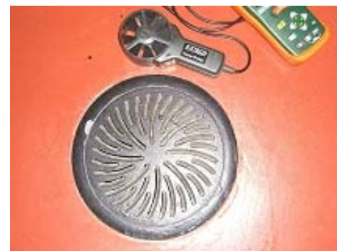
Figure G-38. RAD-3 Underfloor Air Diffuser
