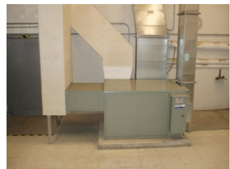
Figure G-51. VRF-2 Air Handler
