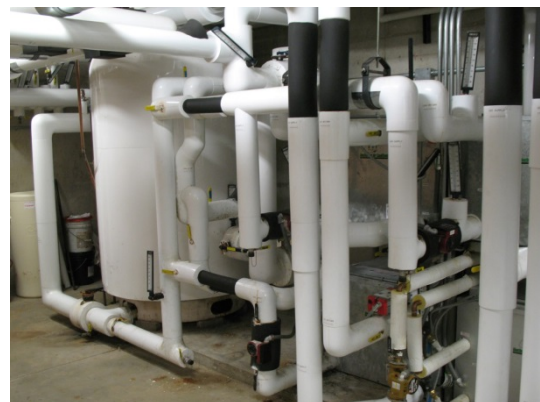
Figure G-31. RAD-2 Heat Pump and Cold/Hot Water Storage.
