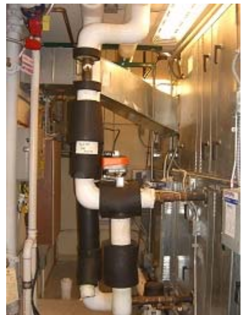
Figure G-36. RAD-3 AHU-3 with Energy Recovery Ventilation Wheel
