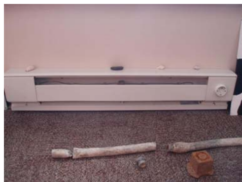
Figure G-58. Typical Electric Baseboard Heater in VRF-2 with Onboard Thermostat.
