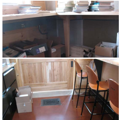
Figure G-30 RAD-2 Diffusers in Offices (On Wall Under Desk) and in Kitchen (in Floor).
