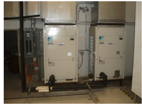
Figure G-52. VRF-2 Air-Cooled Condensing Units
