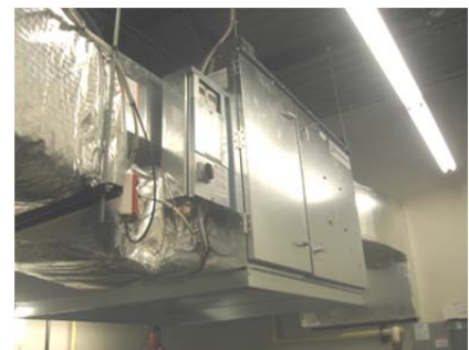
Figure G-61. VRF-3 Energy Recovery Ventilator (ERV-1)
