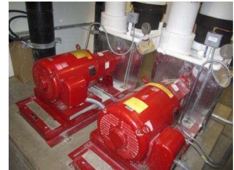
Figure G-8. DV-2 Geothermal Pumps
