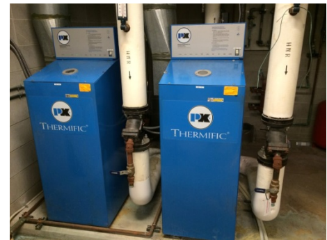
Figure G-17. DV-3 Boilers
