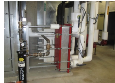
Figure G-24. RAD-1 Radiant Floor HX
