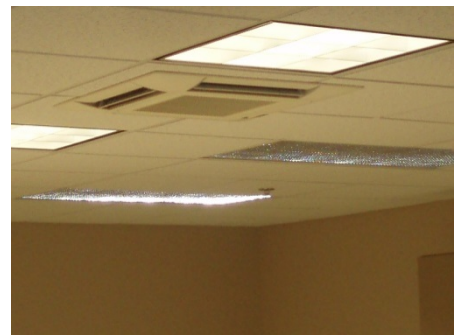
Figure G-53. VRF-2 Ductless Fan Coil Unit
