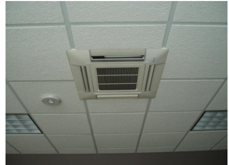
Figure G-43. VRF-1 Ductless Fan Coil Unit
