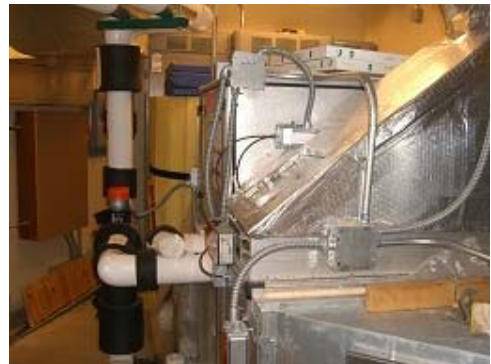
Figure G-37. RAD-3 Air Handler AHU-2
