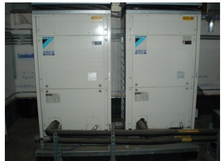
Figure G-42. VRF-1 Air-Cooled Condensing Units
