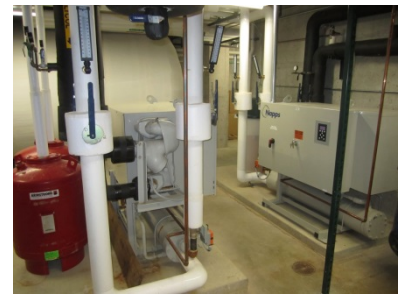
Figure G-23. RAD-1 Chillers
