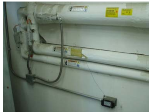
Figure G-57. VRF-2 Domestic Water Piping with Heat Trace and Controls.
