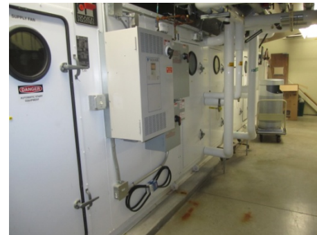
Figure G-4. DV-1 AHU-2 (AHU-3 similar)
