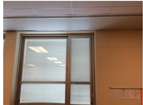
Figure G-16. DV-3 Radiant Heating Panels and Slot Diffuser.
