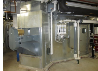
Figure G-22. RAD-1 Air Handler
